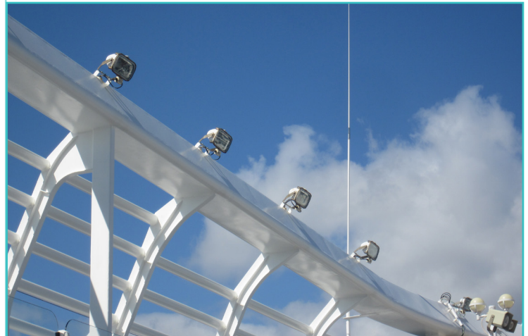
SHIP DECK LIGHTING
